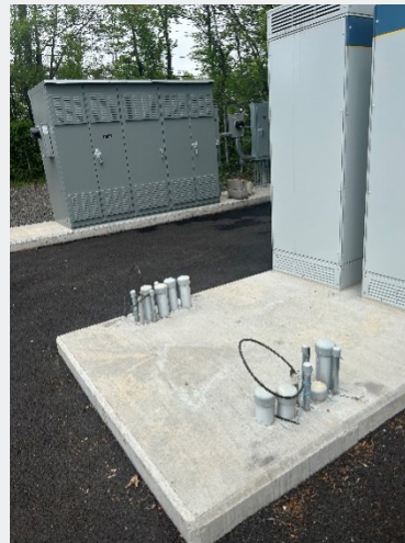
A slab prepared for future EVSE
